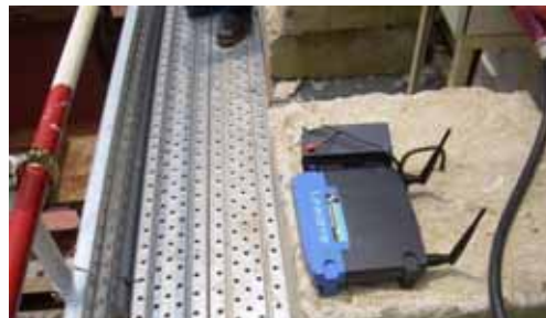
Router 3 placed on concrete slab due to unavailability of mounting surfaces.
