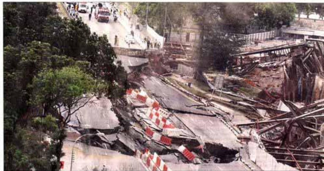
A 30m-deep ravine opened up within minutes of the first collapse, which has initially been blamed on a temporary supporting wall.
